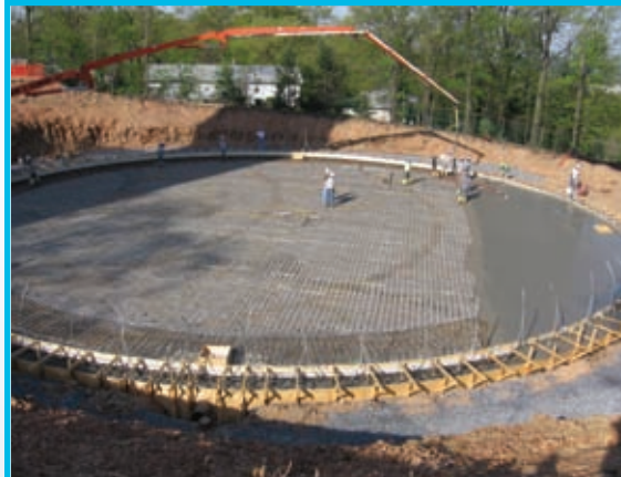
Workers put finishing touches on the base of the new reservoir on Chambers Hill.
